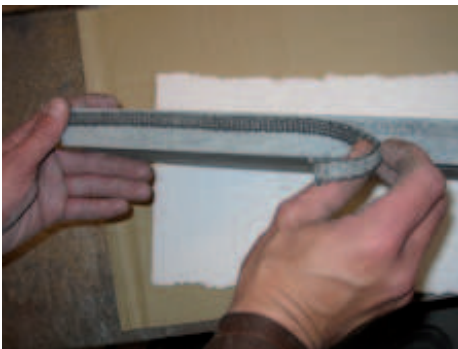
20. Before installing the horizontal stone, attach the sealing strip provided to the back.
